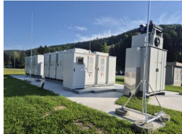
Stromspeicher in Bromberg
